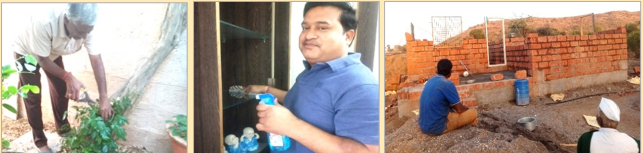
Left to right- B.Bala cleaning the garden, Ravi Singh during the daily chores, Vijay Ukarande constructing a perfect farm house between farms that one can dream of
